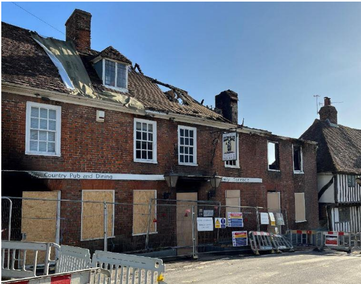
Plate 5. Street View fire damage 2023 (looking South)
